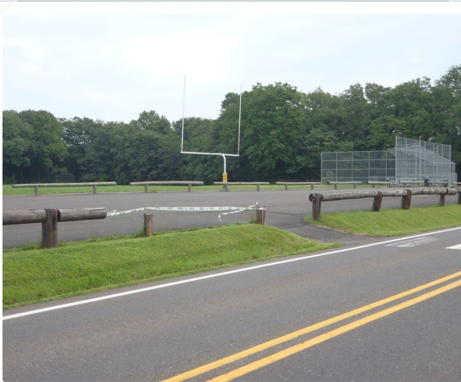
Railings are degraded, broken and missing!
